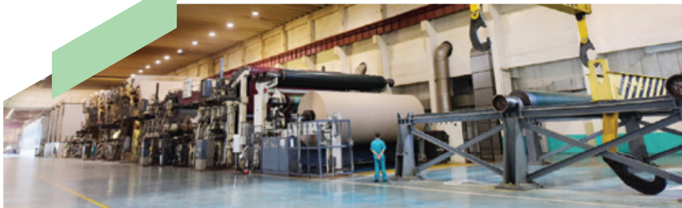
Coated White Top Test Liner production line with an annual capacity of 500,000 tonnes
